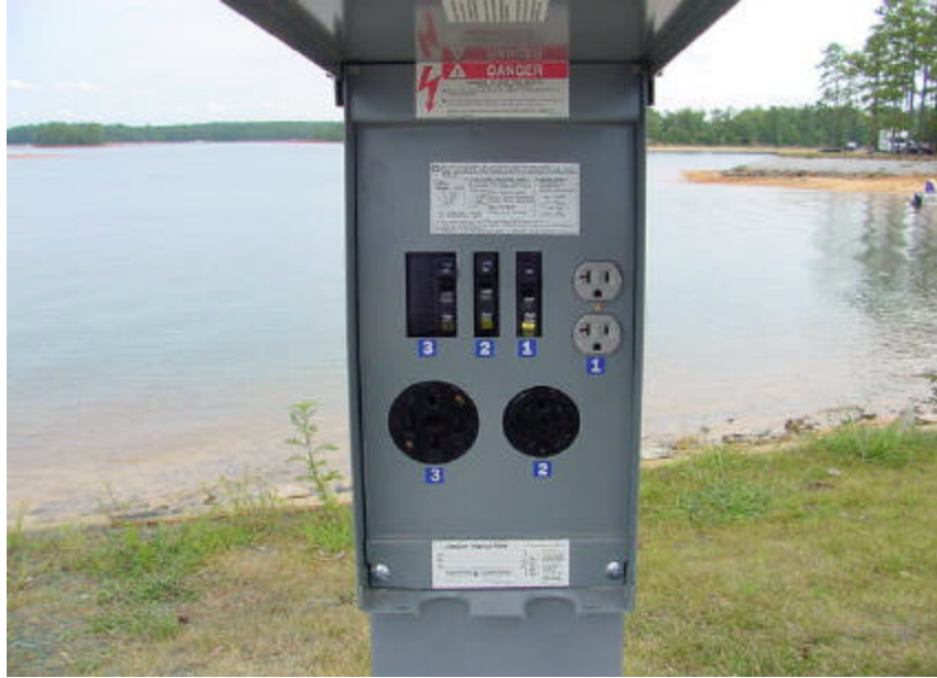
Photo M-15. Electrical Pedestal. Pedestal with 50-, 30-, and 20-amp (GFCI) hookups (Table 5.5)
