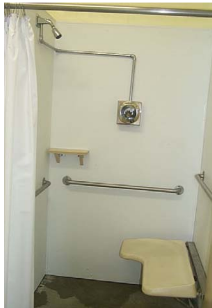
Photo K-8. Shower stall. Redman Creek Campground, Wappapello Lake, MO. Note that a shelf large enough for toiletries is provided in shower stall (Table 3.5). Also note UA rails and bench
